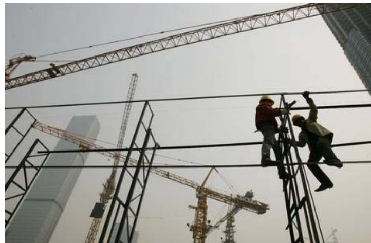
Welders work with no safety harness and no eye protection on a building site in Beijing (Getty)
