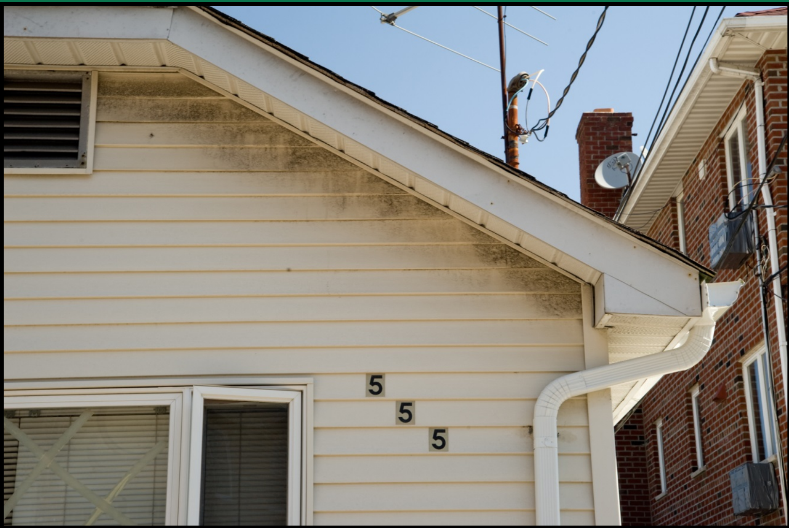
Mold on the exterior of home in Midland Beach. Photo: Karen Smul
